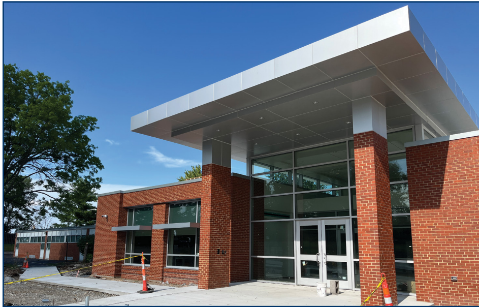
Bierbaum Elementary School has a new secure entrance, reconfigured office space, accessible classrooms and a safer front parking lot configuration. Crews have started work on more classrooms, an expanded library and storm shelter.
